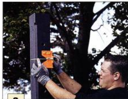
3 Plastic plumb-levelers are attached to the posts and the jig is reintroduced to check for level and proper distance separation.
