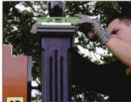
13 To complete the posts we attach finials and caps with silicone being sure that they are level.
