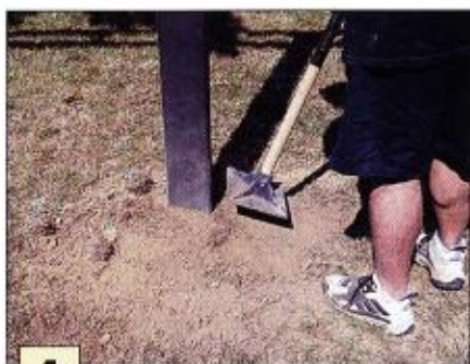
4 The posts are secured with 120 lbs. of dry cement. Eventually ground water will interact with the cement to produce a large pod around each post. When the remaining soil is gathered around each post, it is tamped again with a large 8" x 8" tamper.
