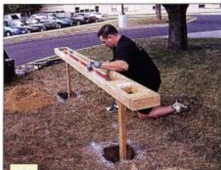
1 Our calibratable installation jig provides numerous assists in the various stages of the installing process. The 10-foot long jig is made of ash to minimize warping. The jig serves as a template for marking the locations where the postholes will be dug.
