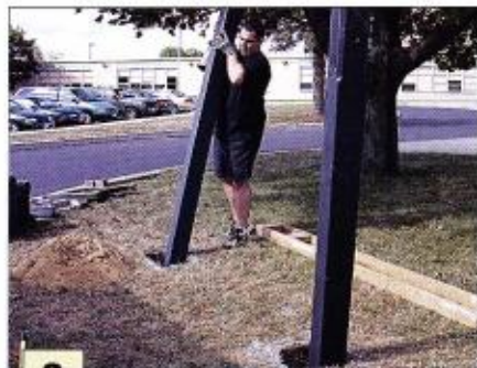
2 The posts are inserted into the postholes. A post leveler in each hole serves to tamper the bottom of the hole and, in conjunction with the jig and a level, determine whether both holes are at the correct depth.
