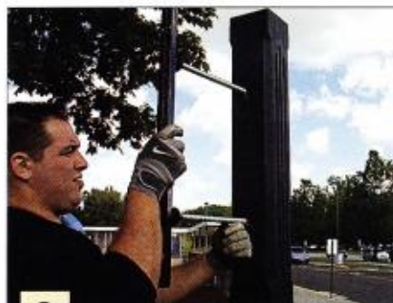
9 Nuts and washers are attached to the threaded rods of the channel brackets before they are inserted into the pre-drilled holes in the posts.
